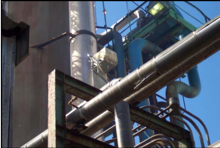
A P2000 installation at Dyno Nobel in Ontario, Canada
