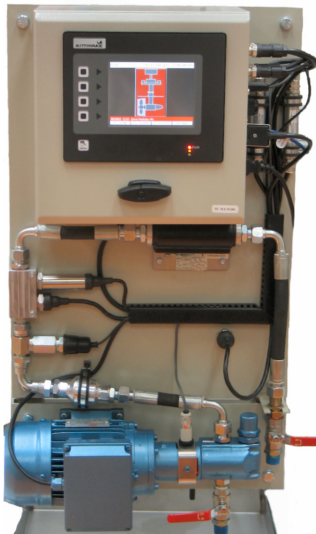
Figure 23 - thruster Monitoring Unit
