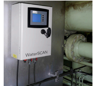
A typical marine installation
